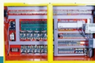
FS-2000D PET 吹拉機電控箱控制系統配置現況 FS-2000D PET BLOWING MOLDING MACHINE OF ELECTROINC CONTROL SYSTEM
